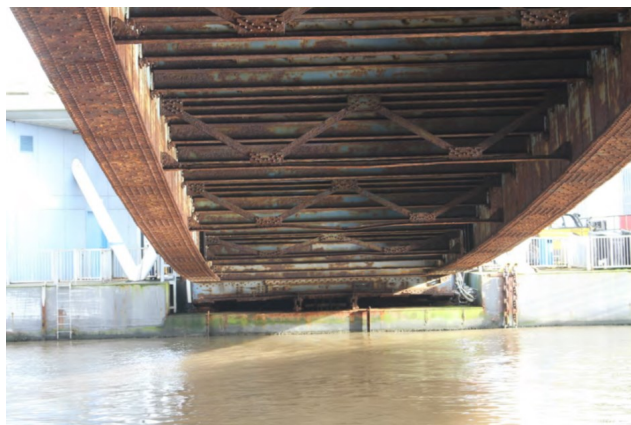
Sub-structure of goods bridge, with bearing mount on pontoon to rear (© Salford Archaeology: Seacombe Ferry Terminal, Birkenhead: Historic Building Investigation)
