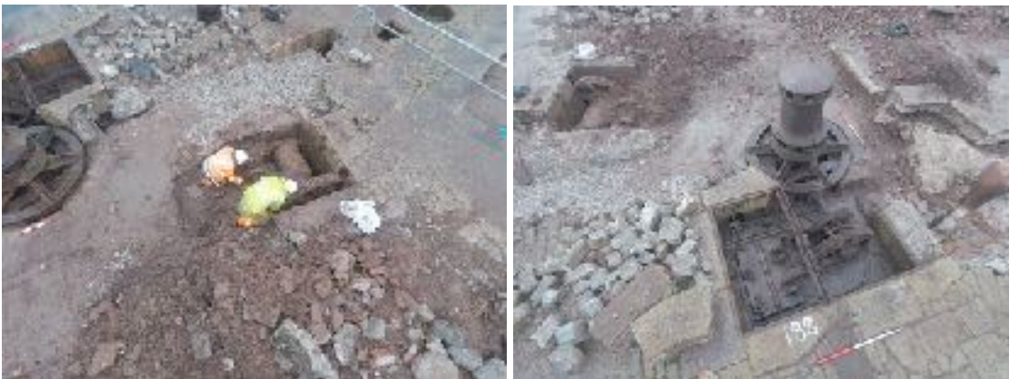
Figure 6. Excavating rubble from a winch used to open lock-gates and a capstan and its hydraulic motors after hand-digging.
