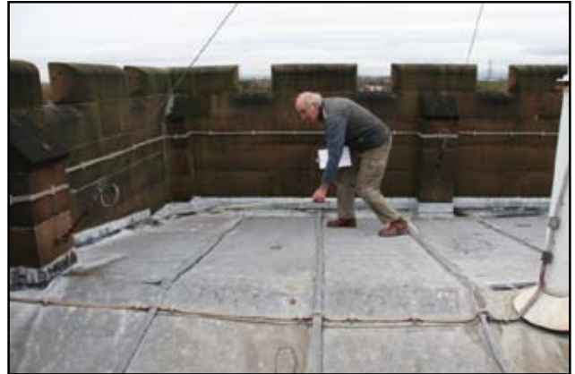
Recording engravings on the lead roof at St Wilfrid's Northenden © Andy Coutts
