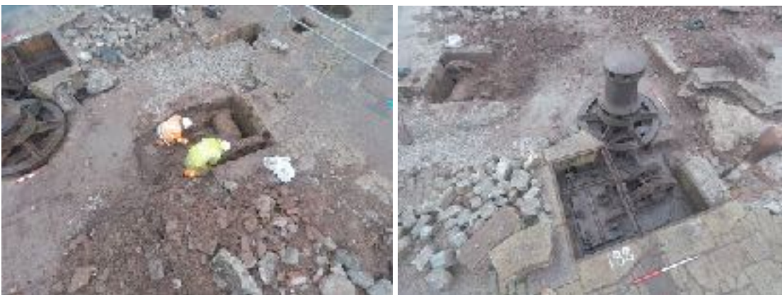
Figure 6. Excavating rubble from a winch used to open lock-gates and a capstan and its hydraulic motors after hand-digging.
