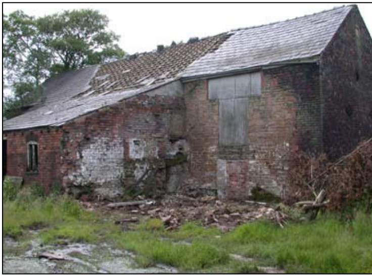
Fig. 2.29: Barn (Building 4) from north-east, showing stone building (Phase A), and outshut (Phase E, to left)
