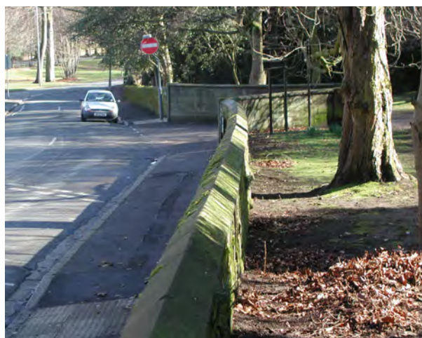
Figure 14. View looking west along Calderstones Park wall showing a curve where it joins the park entrance.
